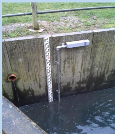
Figure 7-4 Water level monitoring installation in Peterborough
